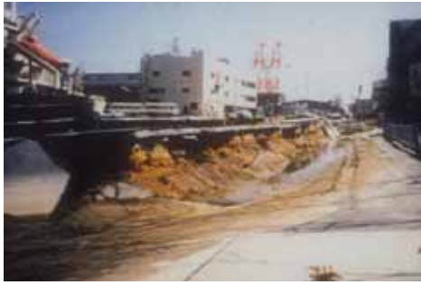
Figure 1: Significant distortion behind a gravity quay wall in Kobe Harbour.
