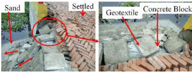
Figure 17 Damages of an approach road of a bridge.
