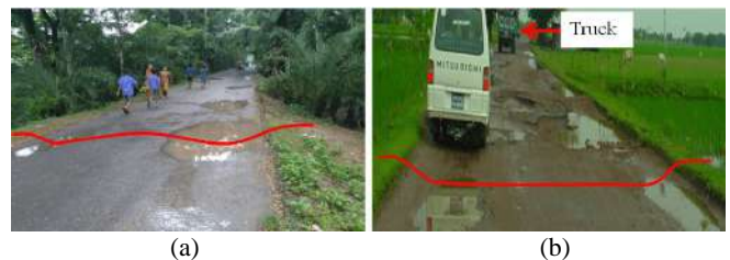
Figure 27 Water logging on the new pavement road. (a) Initial settlement and (b) settlement and wide spread pot holes.
