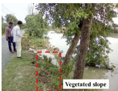
Figure 19 Slope failed in a vegetated slope.
