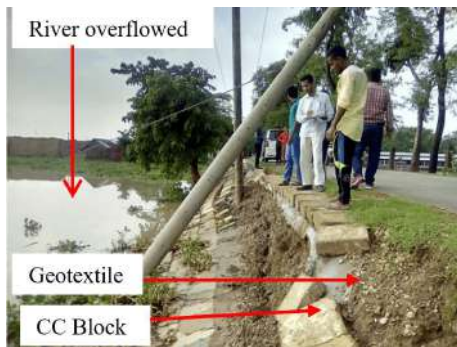
Figure 12 Embankment slope failed.
