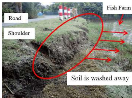
Figure 13 Side slope of rural road washed away by wave action.
