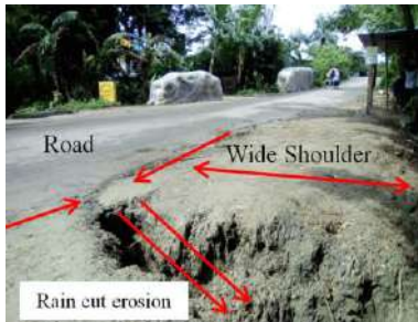
Figure 18 Rain cut erosion in shoulder without vegetation
