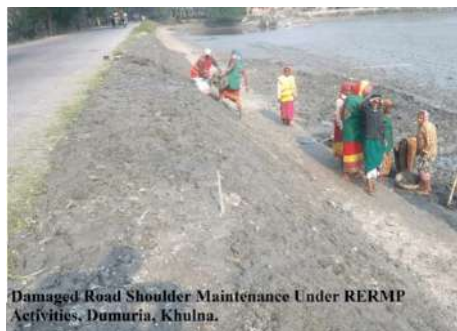
Figure 14 Mud is dumped for repairing side slopes and shoulder (source: LGED website).
