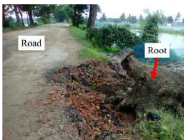
Figure 20 Uplifted tree damaged the road.
