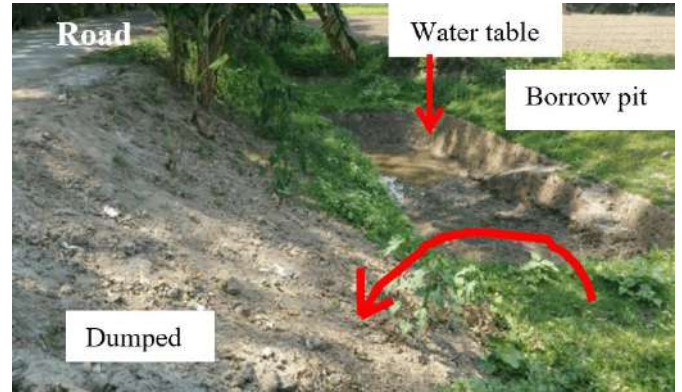
Figure 9 Borrow pit was at the toe of the road. (Location: Babubazar, Barishal).
