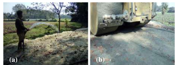
Figure 6 (a) Mixed brick chips and sand (1:1) in Sub-base and watering before rolling and (b) after rolling.
