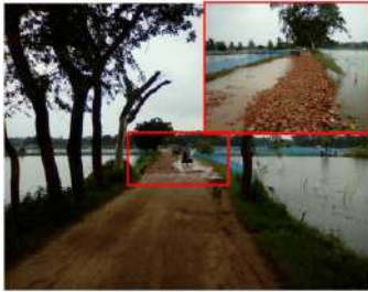
Figure 23 A portion of road settled.
